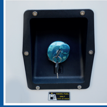
Diesel filling with key lock
