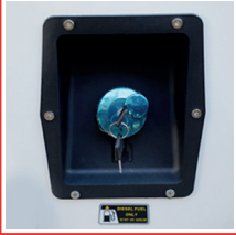
Fuel filling point with key lock
