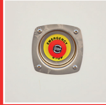
Emergency stop button
